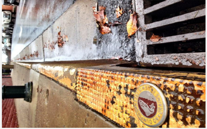
Storm drain in downtown Staunton
